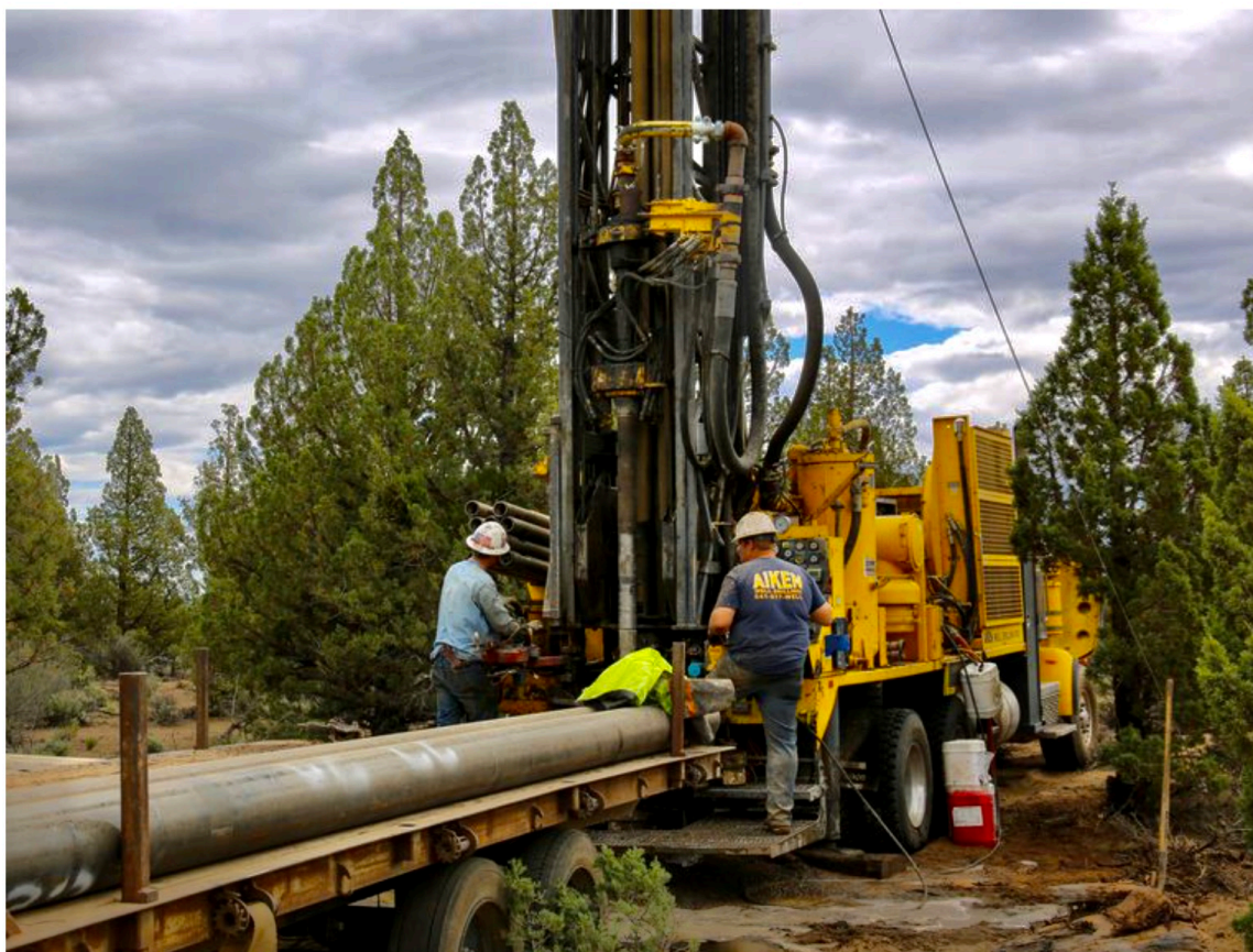
Aiken Well Drilling operators bore a domestic well at a new rural home site about ten miles east of Bend, Ore., July 5, 2022.
